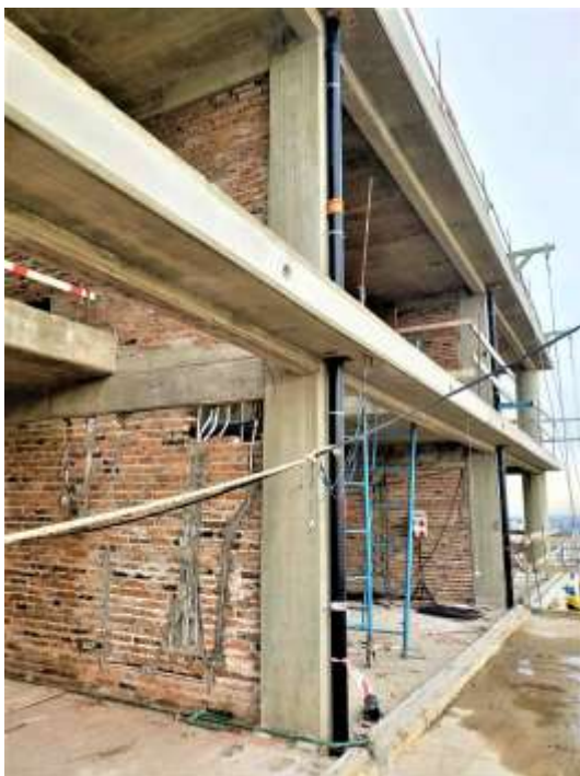
Torre Arcos – 33/34°.P- Inst. Pluvial
